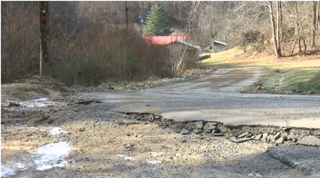
Figure 6-14: 2019 mine blowout damage near Hurley, VA
