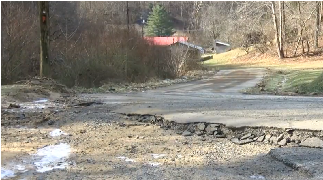
Figure 6-14: 2019 mine blowout damage near Hurley, VA
