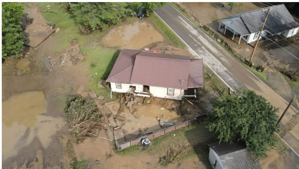
Figure 6-20: Buchanan County home that was pushed off its foundation during July 2022 flooding 34
