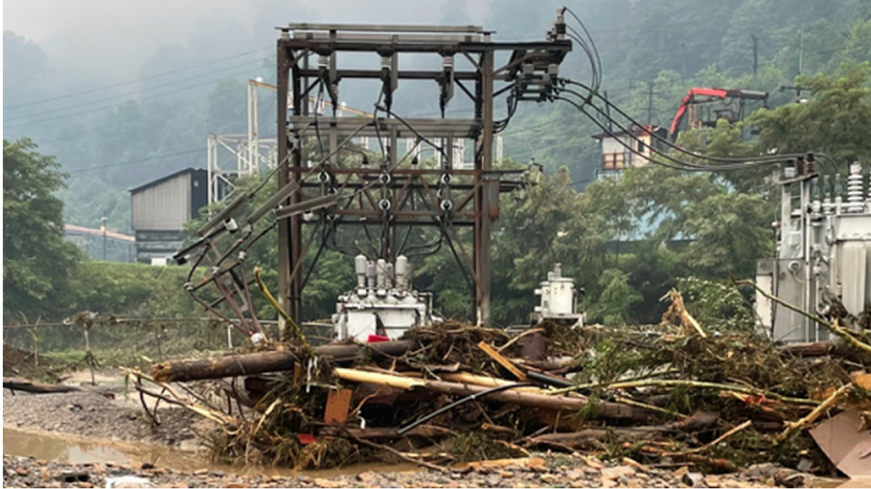
Figure 6-23: Flood damage at Appalachian Power's Dismal River Substation, 2022 37
